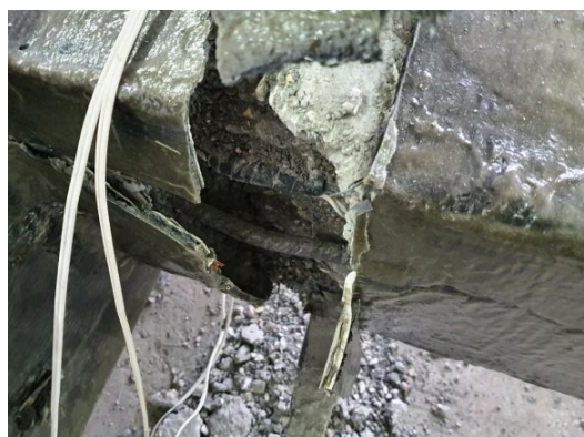
Figure 10. Observed damages during the quasi-static testing of Model M2.
