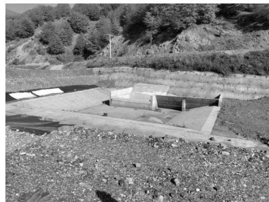
Figure 9. Spillway structure in TSF Sasa 3-2 for evacuation of flood wave from Petrova river
