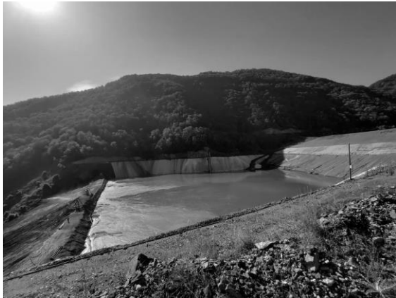
Figure 3. Downstream tailings dam Sasa 4, waste lagoon of Sasa 4, and upstream tailings dam Sasa 3-2. Picture dates from October, 2022
