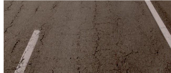
Figure 3. Alligator cracking on the section Velika Kapanica- Babina Greda (left pavement)
