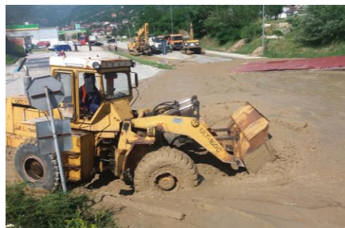
B) Mudflow on the road Tetovo - Jazinec triggered by flash flood of Poroj river (2017 year)
