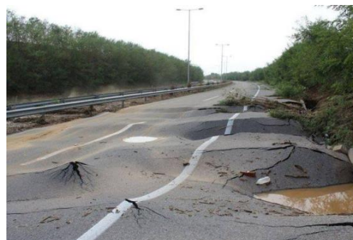
D) Total deformation of the pavement of the northern bypass of the city of Skopje, due to the flood in 2016
