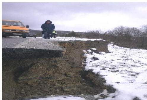
C) Landslide on national road Bitola-Resen (2010 year)
