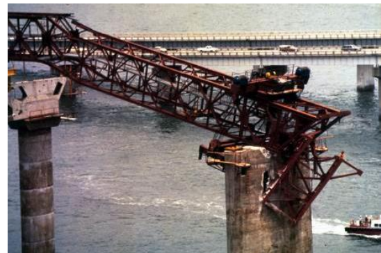
Figure 9. Collapsed construction gantry
