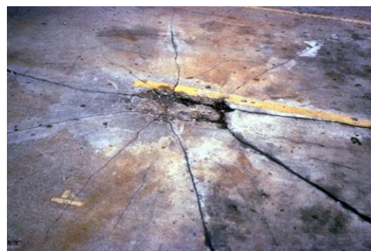
Figure 1. Severely cracked concrete slab
