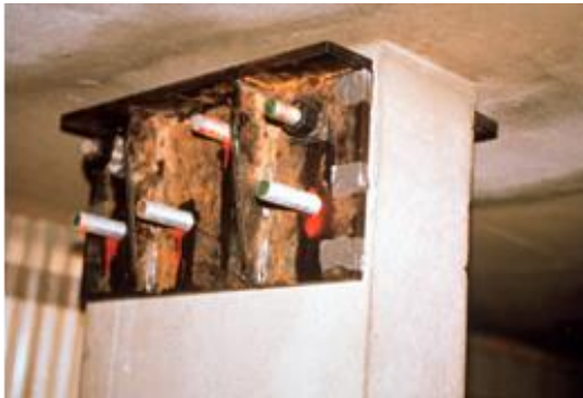
Figure 21. Irregular spacing of anchors
