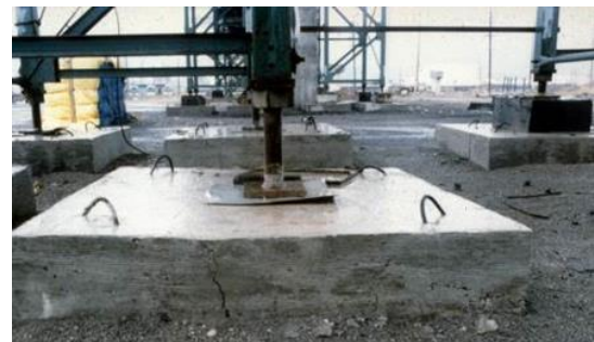
Figure 8. Cracked concrete bearing pad
