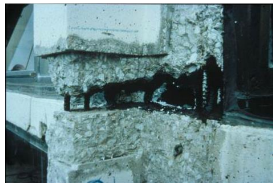
Figure 25. Excessive concrete excavation
