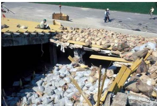
Figure 6. Failure of structure during the load test
