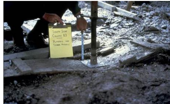
Figure 7. Deflection of shoring mudsill
