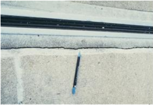
Figure 26. Failed joint seal
