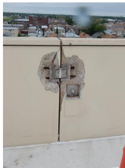
Figure 2. Cracking due to restrained volume change
