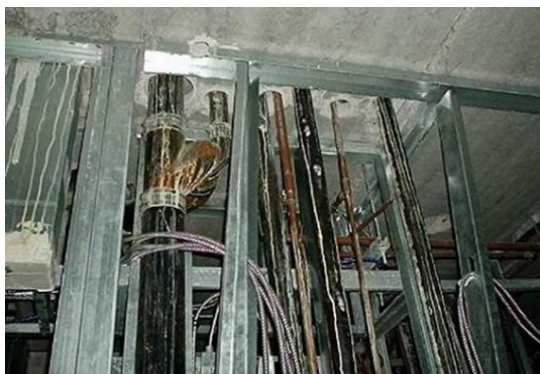
Figure 17. Closely spaced slab penetrations
