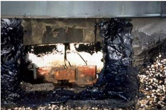
Figure 17. Cracking of panel bearing
