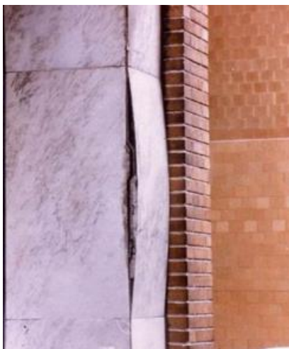
Figure 2. Bowed marble panel due to confined permanent expansion
