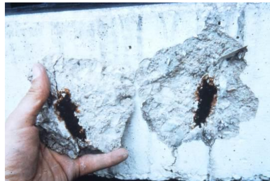
Figure 19. Spalling and cracking of the concrete façade
