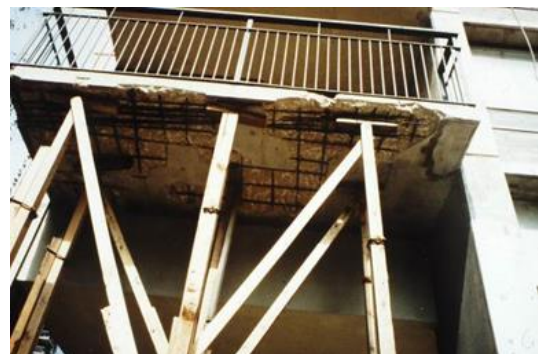
Figure 5. Severely deteriorated balcony requires shoring
