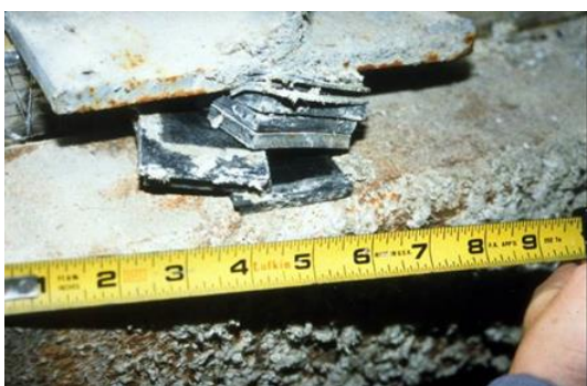
Figure 15. Inadequate bearing of façade panels
