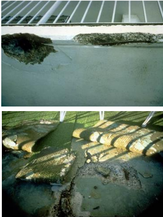
Figure 22. Deterioration of concrete balcony
