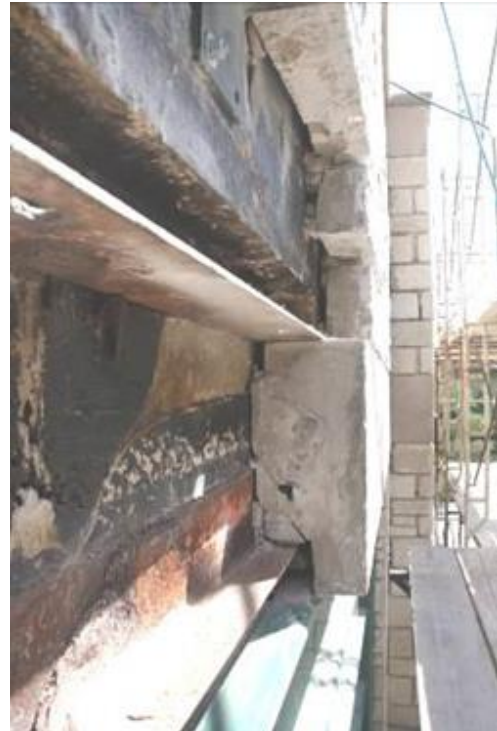
Figure 9. Severely corroded steel shelf angle and cracked and spalled limestone block due to corrosion
