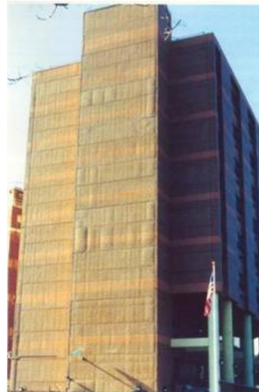
Figure 23. Outward bowing of thin brick bonded to cement board
