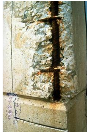
Figure 20. Spalling and cracking of the concrete façade
