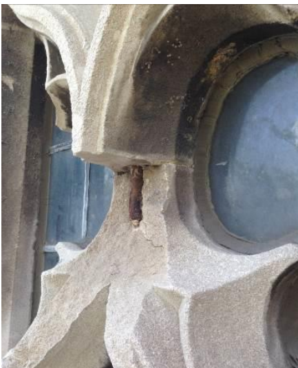
Figure 8. Cracked and spalled window mullions and rosettes
