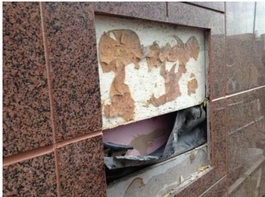
Figure 10. Granite inserts attached with epoxy adhesive that has failed
