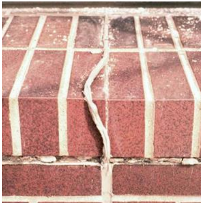
Figure 1. Moisture expansion of brick
