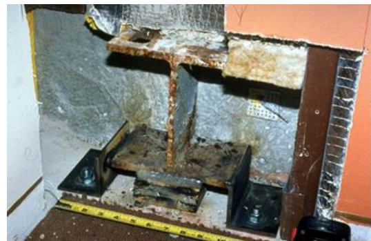
Figure 16. Typical gravity load connection repair
