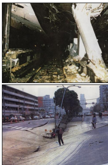
Figure 2. The seismic damage of the Daikai subway station (above) and the road subsidence above the station (below) [13]
