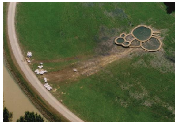
Figure 7. Piping (soil boiling) far away from the dyke and stabilizing measures to reduce the hydraulic gradient (photo: L. Nagy)
