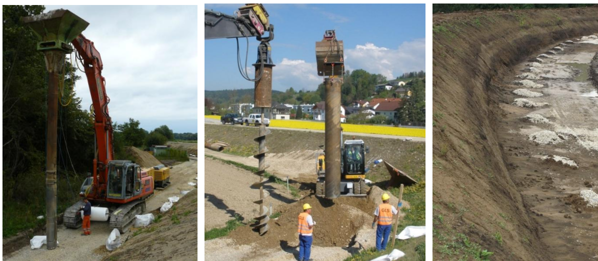
Figure 15. Installation methods of relief drainage columns wrapped in nonwoven geotextile. (left: vibroflotation method; middle: rotary drilling method with casing; right: “infinite” relief column system at the dyke toe)
