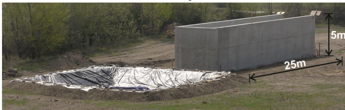
Figure 22. The large scale test facility (length 25 m, height 5 m und width 4 m) for investigating the underseepage of dykes and levees in a 1:1 scale
