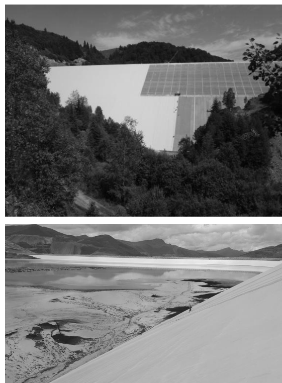
Figure 5. Geocomposites on extruded curbs: at left Runcu GFRD in Romania, at right a tailings dam in South America
