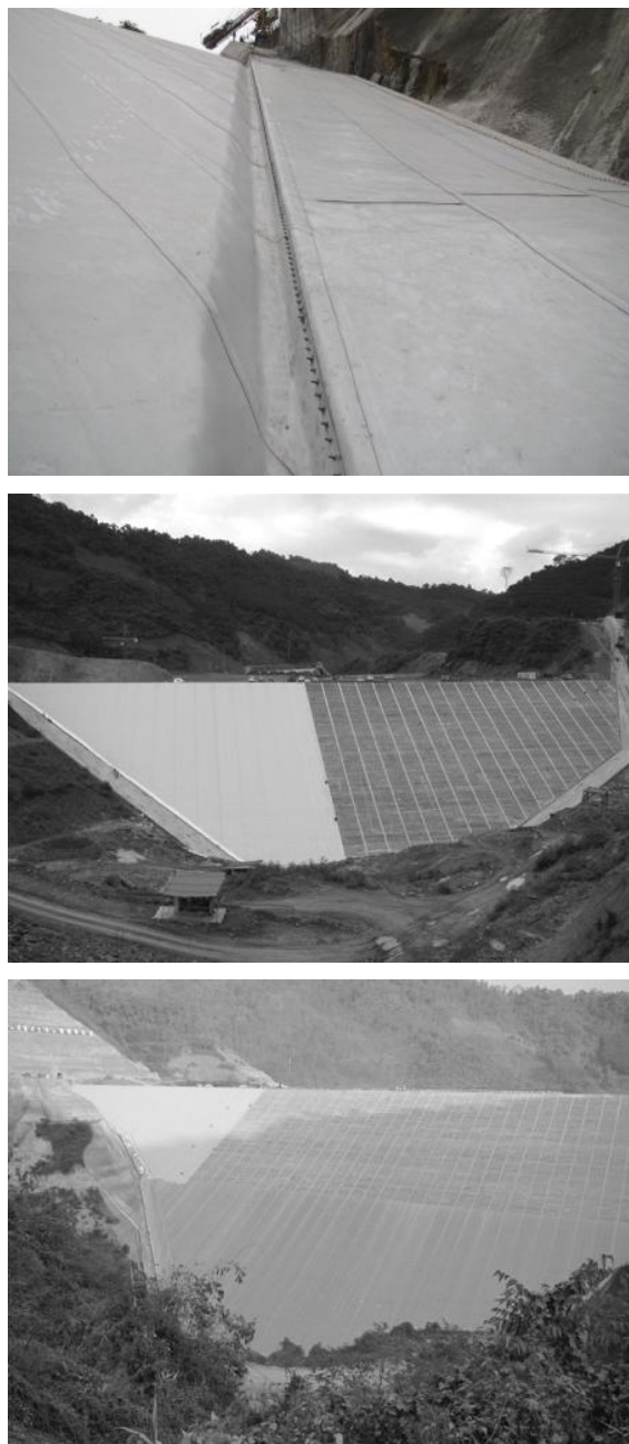
Figure 4. Nam Ou VI GFRD: Watertight perimeter seals at plinth, and Stage 1 and Stage 2 waterproofing
