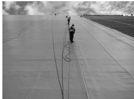
Figure 3. Nam Ou VI GFRD: Seaming of SIBELON® CNT geocomposite to anchor strips and of adjoining geocomposite sheets
