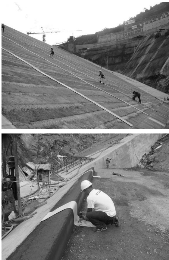
Figure 2. Nam Ou VI GFRD: The SIBELON® PVC anchor strips placed on the extruded curbs
