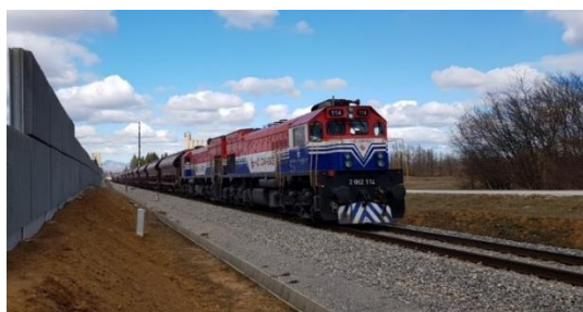
Figure 12. First application of RUCONBAR noise barriers on railways line (noise protection of the settlement near railways station Gospić)
