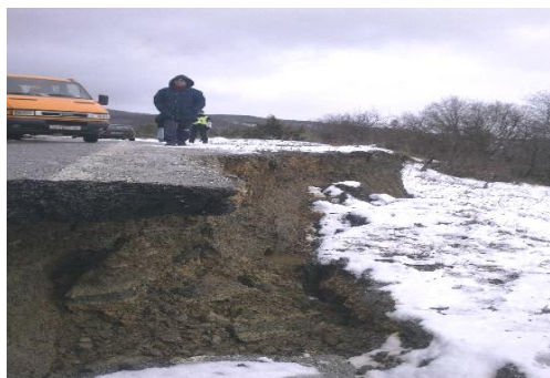
C) Landslide on national road Bitola-Resen (2010 year)
