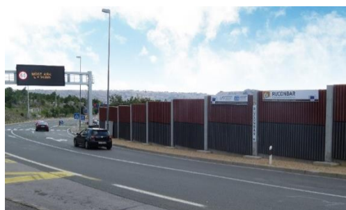
Figure 11. First application of RUCONBAR noise barriers on road section (noise road protection of the settlement Scott)
