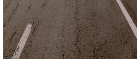
Figure 3. Alligator cracking on the section Velika Kопanica- Babina Greda (left pavement)
