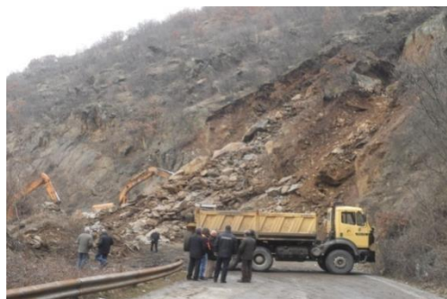
A) Rockfall on the road Istibanja – Makedonska Kamenica (2015 year)
