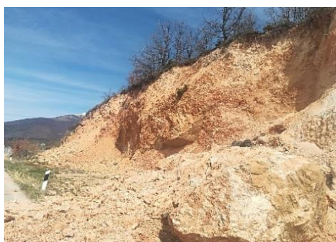
G) Landslide on the road Resen – Greece Border, place Markova Noga, in 2017
