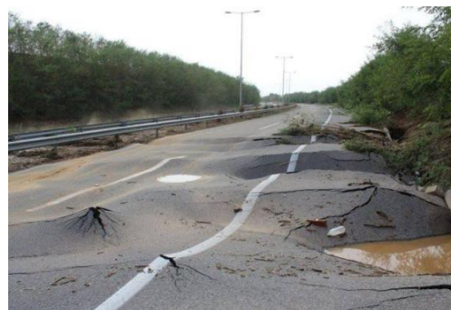
D) Total deformation of the pavement of the northern bypass of the city of Skopje, due to the flood in 2016
