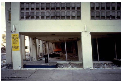
Figure 1. Soft-story mechanism in the ground floor
