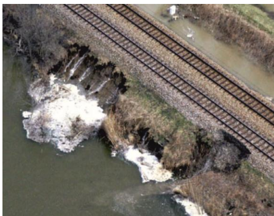
Figure 6. Piping through a railway embankment during an already sinking flood. Train traffic was stopped
