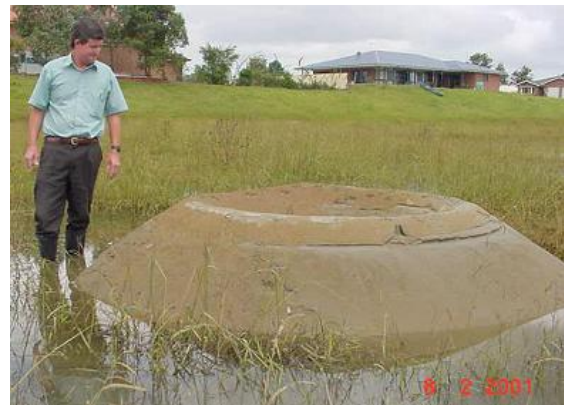
Figure 8. Boiling “volcanoes” after the flood. Retrogressive internal erosion towards the dyke causes stability loss in the long-term (photo: L. Nagy)
