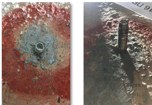
Figure 9. Failure of anchor type 1
