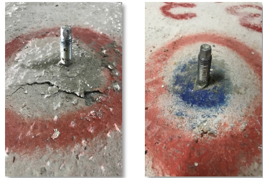
Figure 11. Failure of anchor type 3
