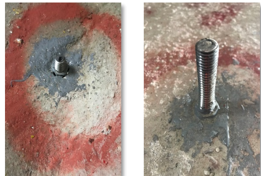
Figure 12. Failure of anchor type 4
